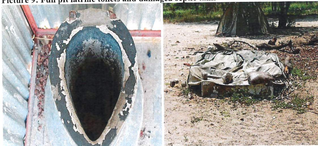
Picture 9: Full pit latrine toilets and damaged septic tank
